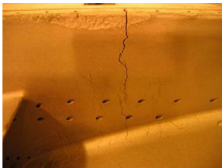
Fig. 6 1.5 mm wide cracks on the sidewalls of a typically industrial gas turbine nozzle segment
